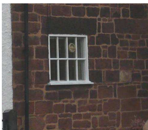
No 6 The Rake: A wooden replacement window in the spirit of the original but with a protruding cill and an extractor fan inappropriately placed. Its slightly awkward appearance suggests the original window may have had 12 panes rather than 8.
