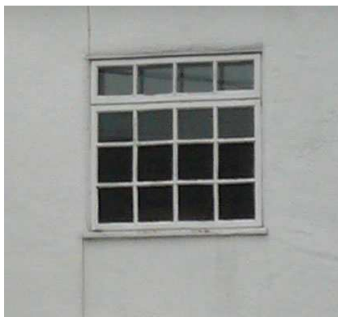
No 26 Bromborough Village Road: although the lights are appropriately sized, the square window openings now contain top hung casements, which are out of character
