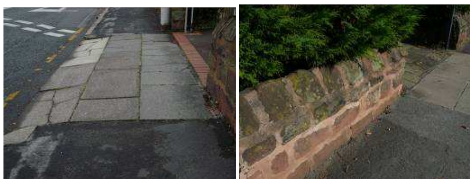
Poor quality surface treatments do little to enhance the setting of the conservation area
