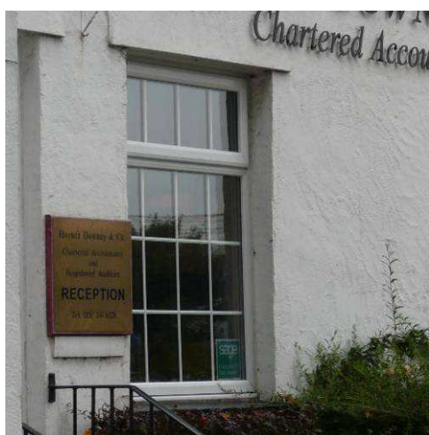
No 28 Bromborough Village Road: the openings originally would have been fitted with sliding sash windows, probably 8 panes over 8 and although an attempt has been made to emulate the historic glazing pattern, the use of uPVC top-hung casements has resulted in windows with ungainly proportions
