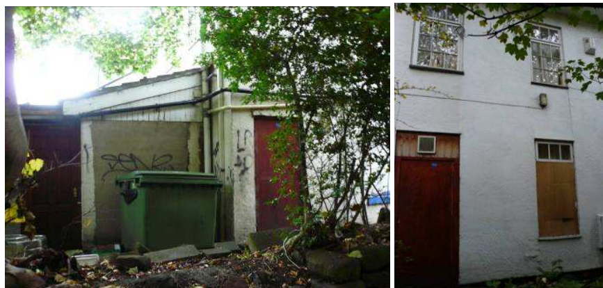
The rear of Nos 32-34 Bromborough Village Road sits alongside the pathway to the church and is in need of some improvement
