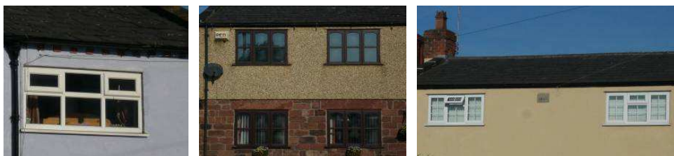
Small rectangular openings at Nos 8, 10 and 20 The Rake (unfortunately fitted with replacement windows)
