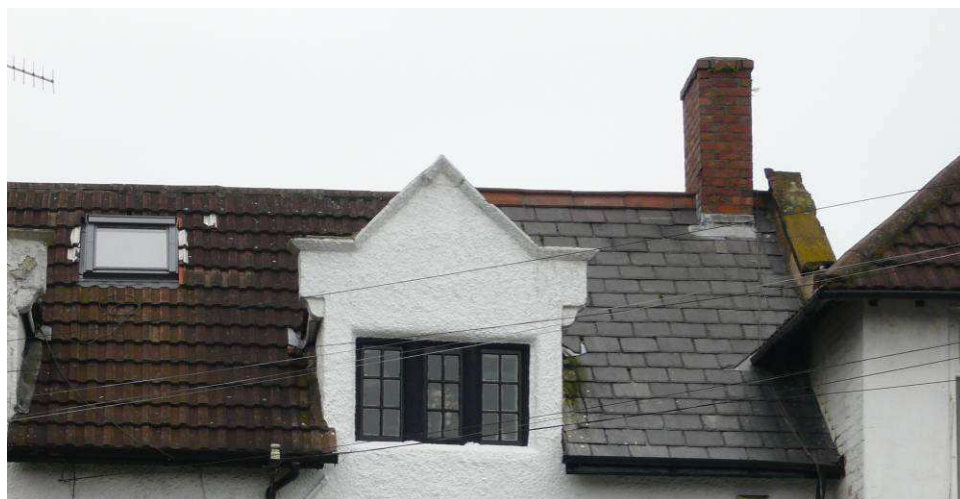
Nos 54/54a Bromborough Village Road demonstrates the difference in appearance between a slate roof (right) and modern interlocking profiled tiles (left)
