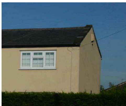
No 20 The Rake: The outer lights have side-hung casements and the central one a small top-hung casement, a feature alien to the original form of such cottage windows. Each light has imitation glazing bars sandwiched between the panes of glass. If the window openings are original, they would have most likely contained a three-light window with a central side-hung casement. The cluttered design of these windows does little to preserve or enhance the character of the building.
