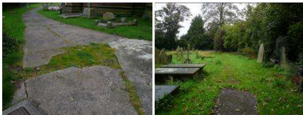
(left) The concrete pathways within the churchyard are in need of repair or replacement and do not enhance the setting of the church. The pathways turn to grass towards the northern end of the churchyard, making them uninviting and potentially dangerous in wet weather (right).
