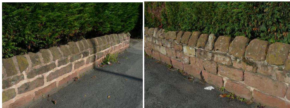
Different treatments of sandstone walls to neighbouring properties
