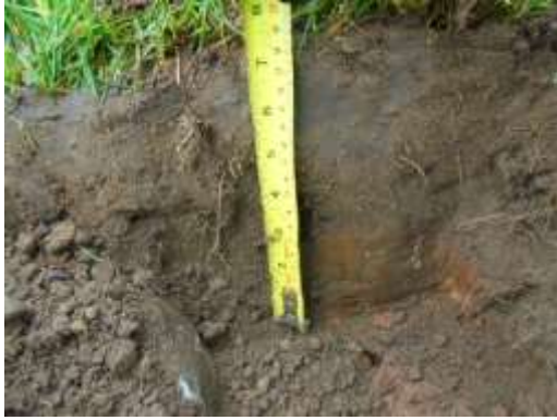
Plate 5: Example of the 1994 system capped by topsoil and the backfill heavily contaminated
