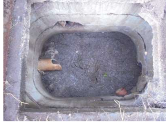
Plate 6: Inside the existing inspection chamber which requires replacement due to its condition. Note the build up of silt in the base of the chamber
