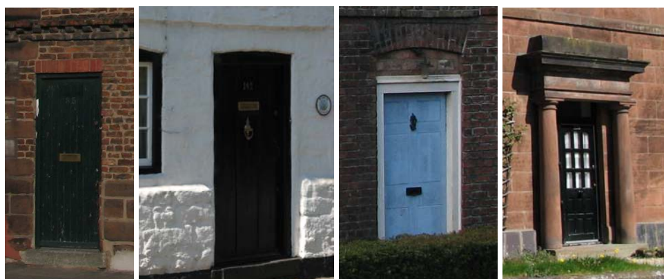
Doors and door surrounds in the conservation area. (1) and (2) are simple boarded doors, (3) is a 6 panelled door, probably altered slightly from its original arrangement. (4) is the classical door surround to The Old Post Office with a modern door.
