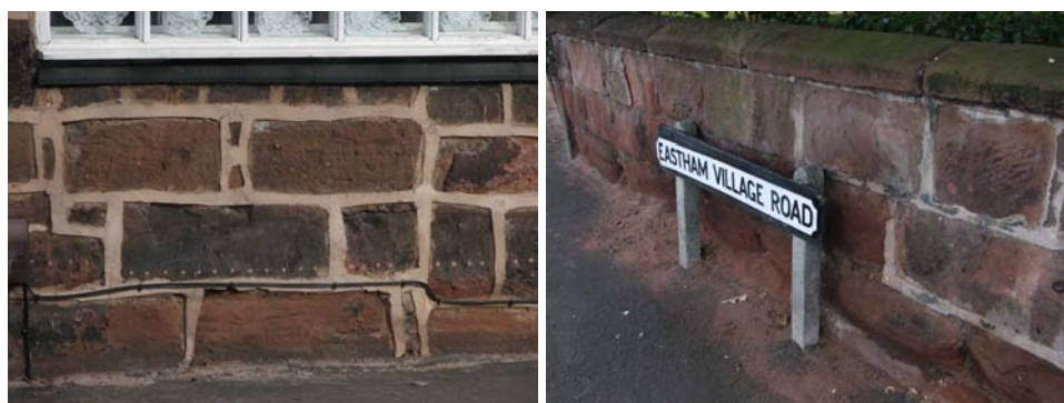
(left) the visually detrimental effect of the insertion of an injected damp proof course and poor quality pointing; (right)
