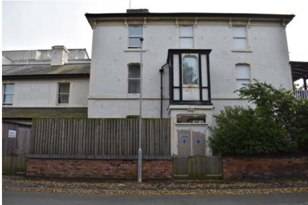
4.3.7 Valentia Road elevation of the former hotel with deteriorating fabric
