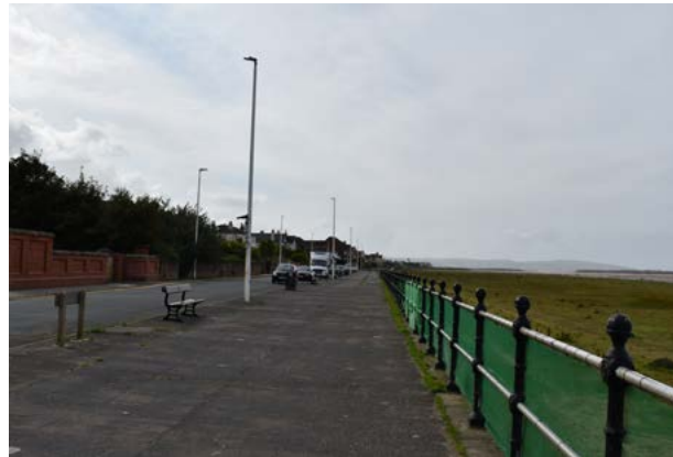
4.6.11 Promenade with deteriorating tarmac
