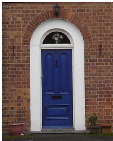
Fine and authentic, deeply panelled mid-Victorian door on The Village; now sadly replaced by a standard unit, lacking the original's individuality.
