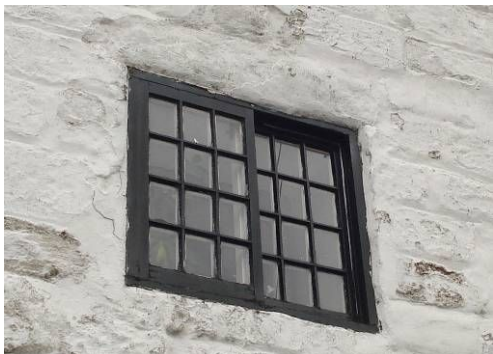
C17th-18th small paned, horizontally-sliding sash, Leaded light in the same property to first floor of Willow Cottage.
