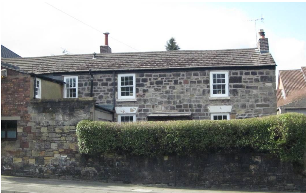
No. 32 Heath Road – traditional C17th vernacular stone cottage. Vertical sash windows were probably added in the early C19th; traditional timber sashes recently reinstated.
