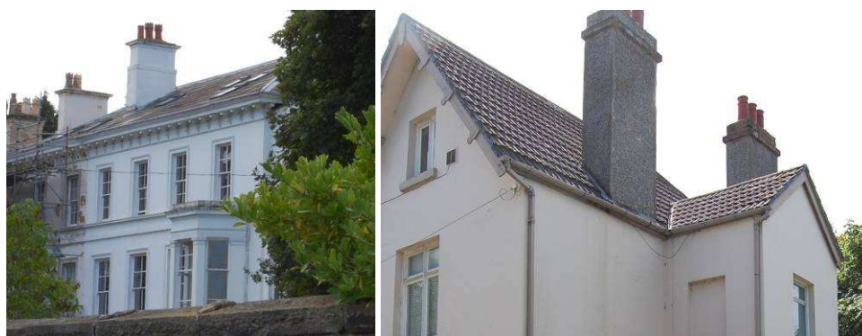
Unsympathetic alterations within the conservation area: (left) rooflights inserted into the roof slopes; (right) concrete pantiles
