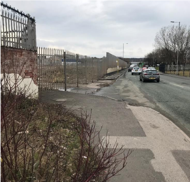
Figure 17: Poor quality foot way at Wallasey Bridge Road
