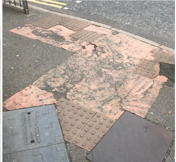
Figure 18: Degraded pedestrian crossing at Poulton Bridge Road
